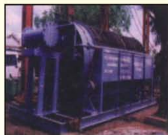
Blow Down Tank
