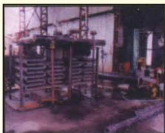
Steam Distribution Header
